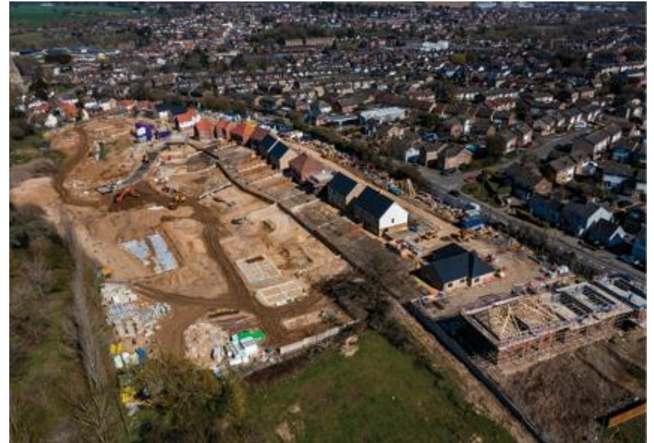
New homes under construction in Halstead. Thousands of new homes are expected to be built each year across Essex. Until a reliable and well-tested version of the Home Energy Model becomes available, an affordable interim tool is required that can provide realistic predictions of energy performance to ensure planning applications for new homes can reliably demonstrate performance against net zero policy requirements.
